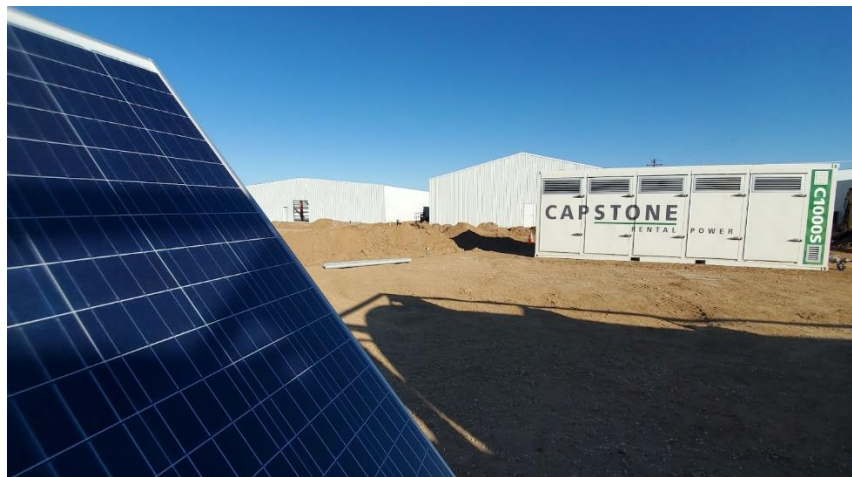
CAPTION: Instant ON Microgrid Gap Solutions in California City leverage on-site turbines, batteries, solar and fuel cells.
