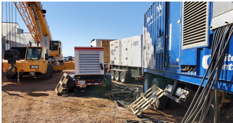
CAPTION: Before the Instant ON Microgrid Gap Solution replaced these three diesel generators.
