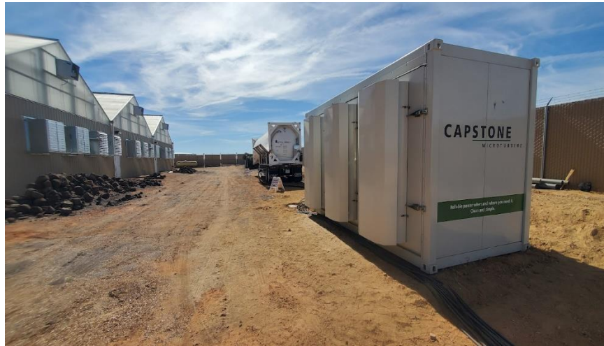
CAPTION: After the Instant ON Microgrid Gap Solution replaced three diesel generators with a single unit, freeing up valuable space, eliminating dangerous exhaust fumes, and making the area more presentable.
